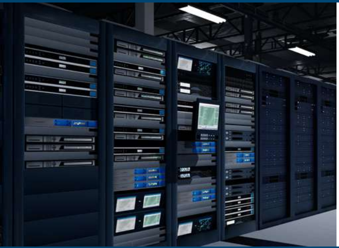
MNL1 Data Center, Philippines IFC EDGE
